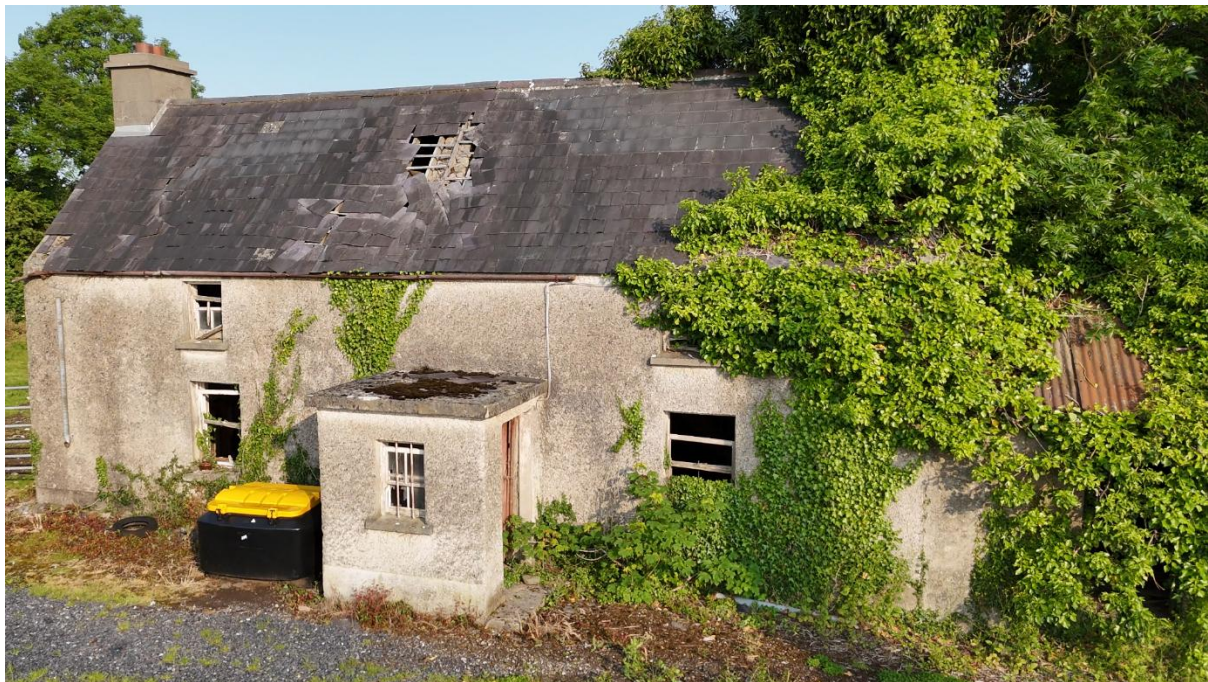
Figure 2.5 Photograph of derelict dwelling to be demolished
