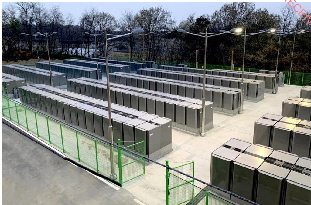
Figure 2.20 Modular Energy Servers positioned at ground level 9
